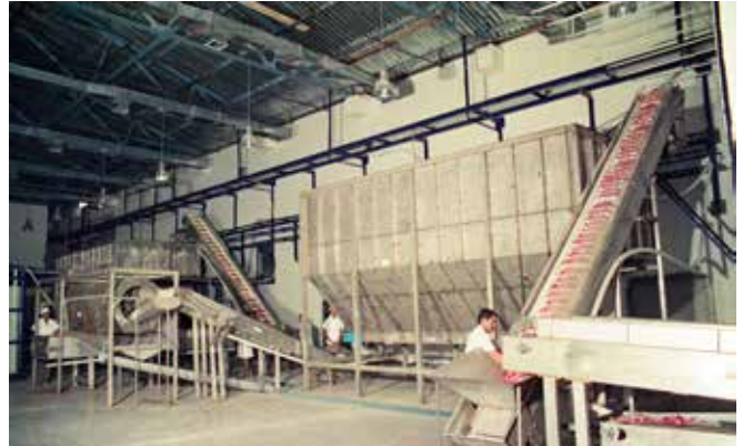
View of the largest Onion and Vegetable Dehydration plant in the India.
